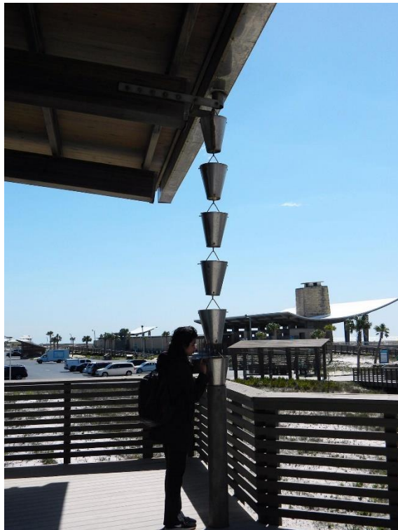
Figure 5. Decorative rain chains help direct rainwater into the cistern (LeBleu, 2022).
